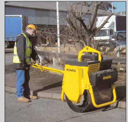
Standard with water sprinkler system.
